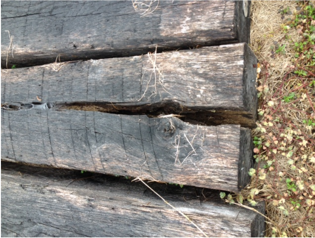
Figure 7 - Tie #249 (unt. red oak) with severe split and decay fruiting bodies on end grain.
