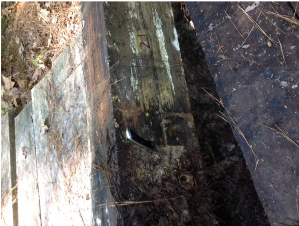
Figure 4 – Tie #21 (unt. red oak) tie with light decay.
