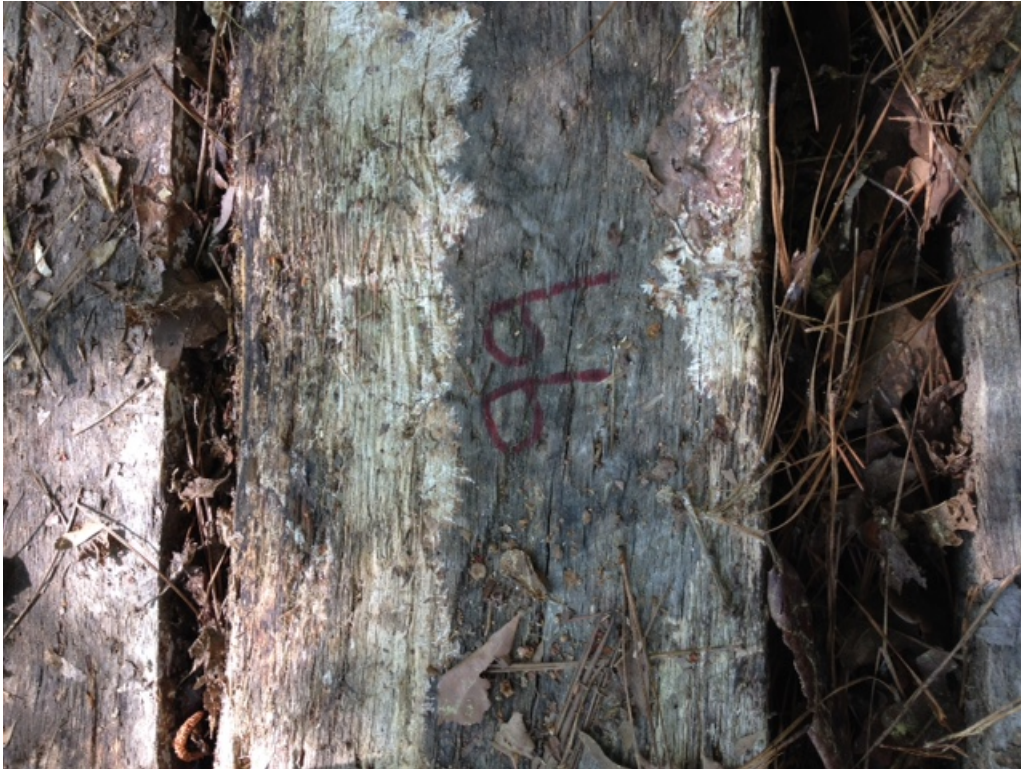
Figure 3 - Tie #99 (unt. white oak) showing trace amounts of decay.
