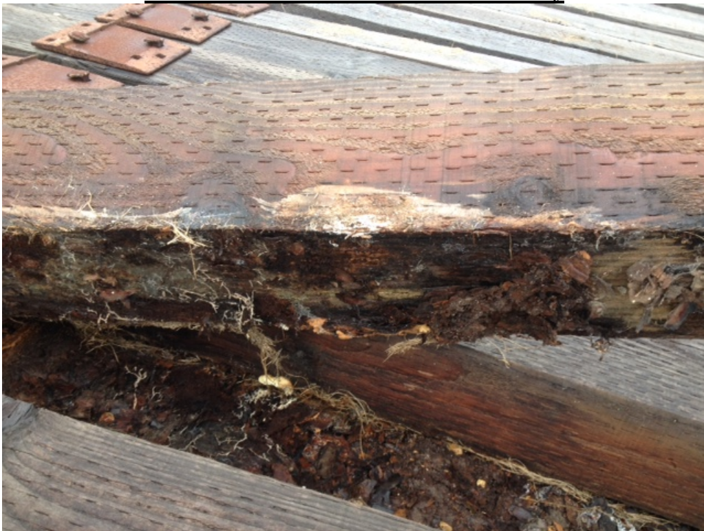
Figure 6 - Tie #106 (unt. D-fir) with visible decay.
