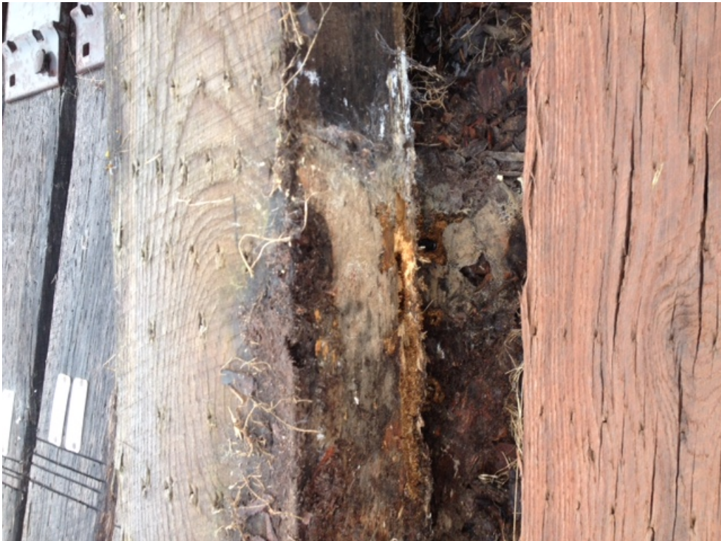
Figure 8 -Tie #40 (unt. white oak) with decay and beetle damage.
