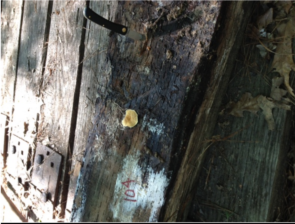
Figure 5 - Tie #104 (D-fir untreated) with light decay.
